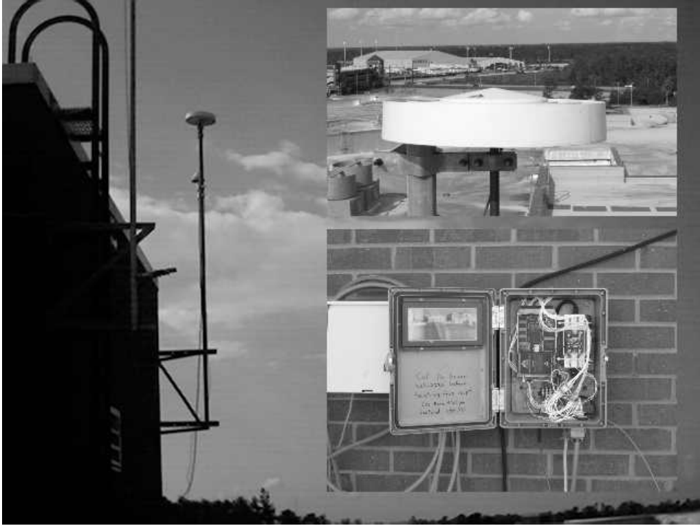
Figure 45 – GPS Antenna on Mast
