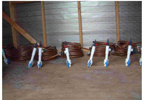
Figure 3-3 Effluent Standpipes, Coupon Cradles and Corrosion Loops
