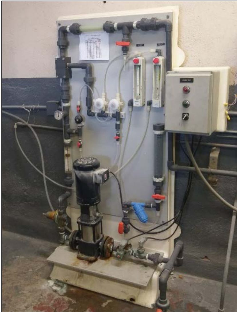
Figure 4-2: Evoqua® ClO 2 Generator (Harry Simmons WTP, Griffin, GA)
