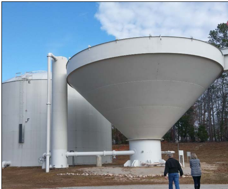
Figure 3-2: ClariCone ® Solids Contact Unit Located At Emerson L. Burford WTP
