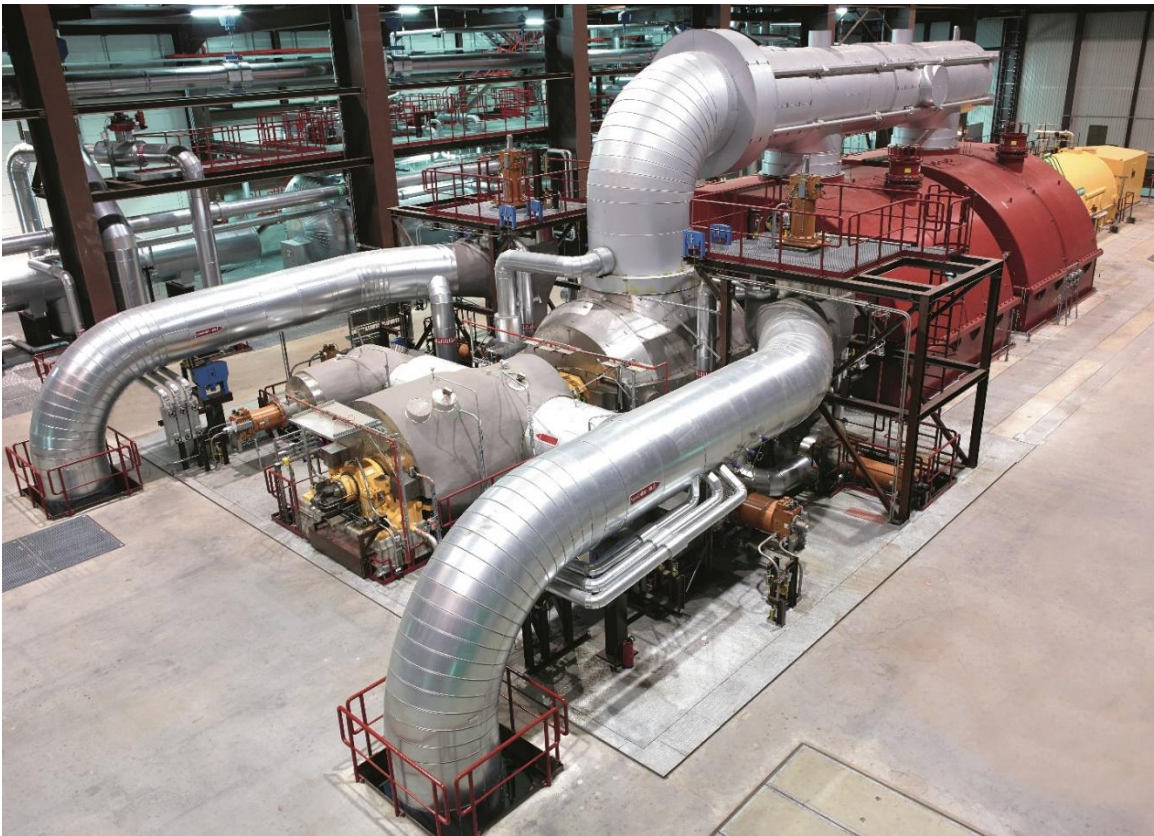
Figure 2.9: Siemens SST-6000 steam turbine in Lünen Power Station, Germany
